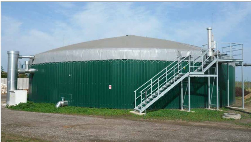
Figure 3: Anaerobic digester converting spent mushroom substrate into biogas, heat and fertilizer (Source: László Somos).
